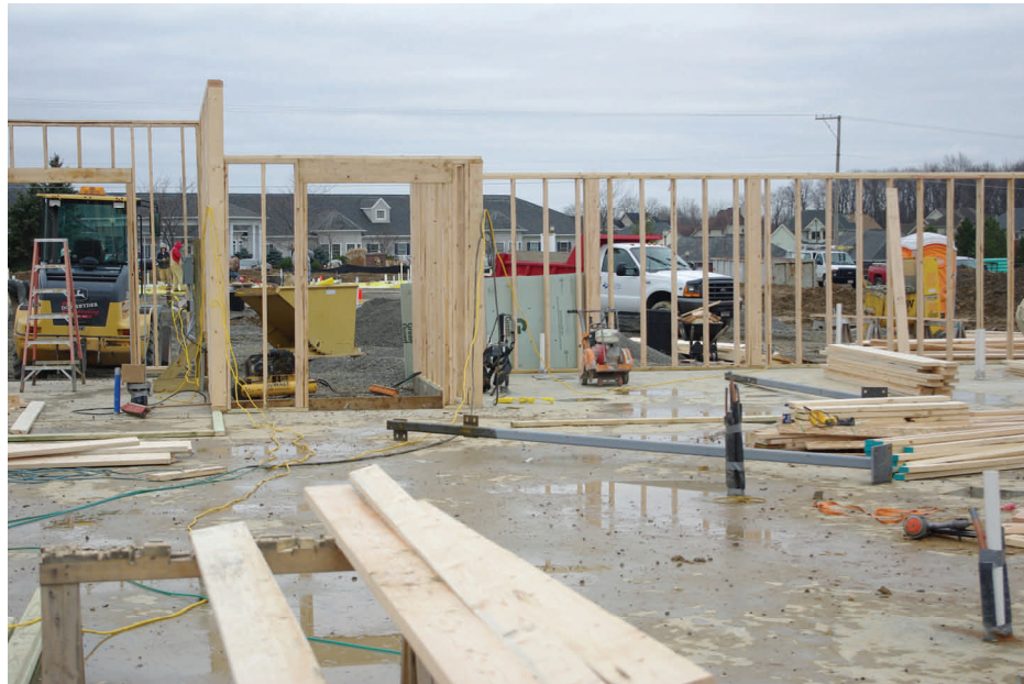
Garlock Brothers Construction based in Findlay, OH has made steady progress on the Green House homes in spite of record rainfall.
